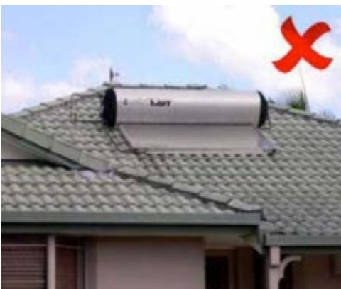
Solar heating visible from street
